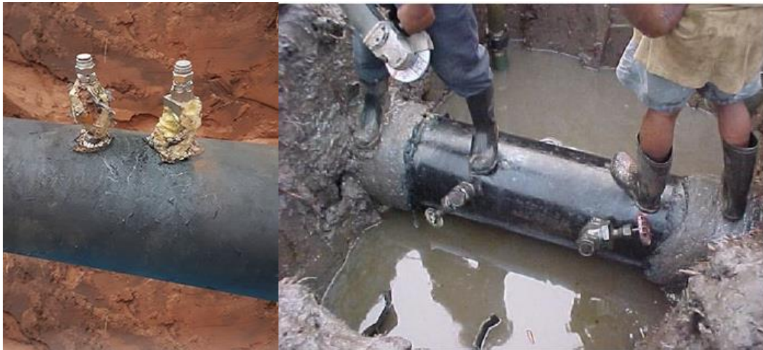
Figura 4.6 Tomas ilegales en ductos. Fuente: Tomada de Hot Tapping and Product Theft from Pipelines. A Way to Detect and locate these Spots during Normal operation, Pipeline Technology Journal. Issue 1. P. 26. 2017 www.legaloil.com/Images.asp
